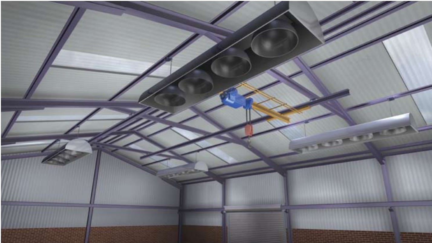
Hanging of industrial lighting systems
